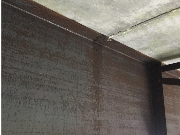
Minor corrosion noted at deck joints
